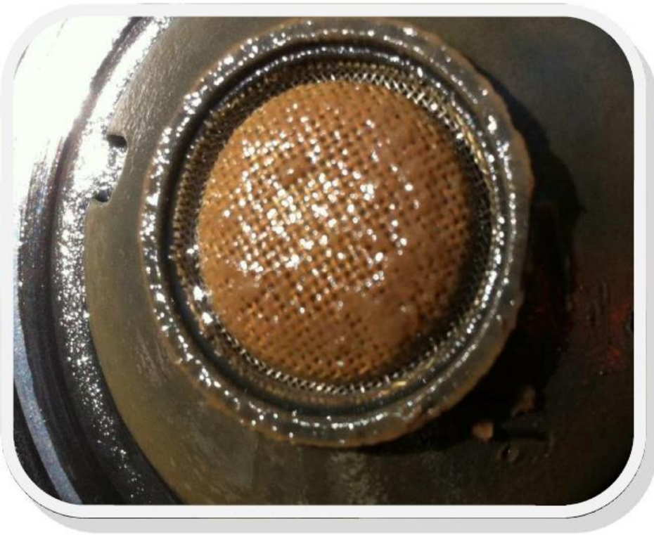
Irrigation Valve Filter before
